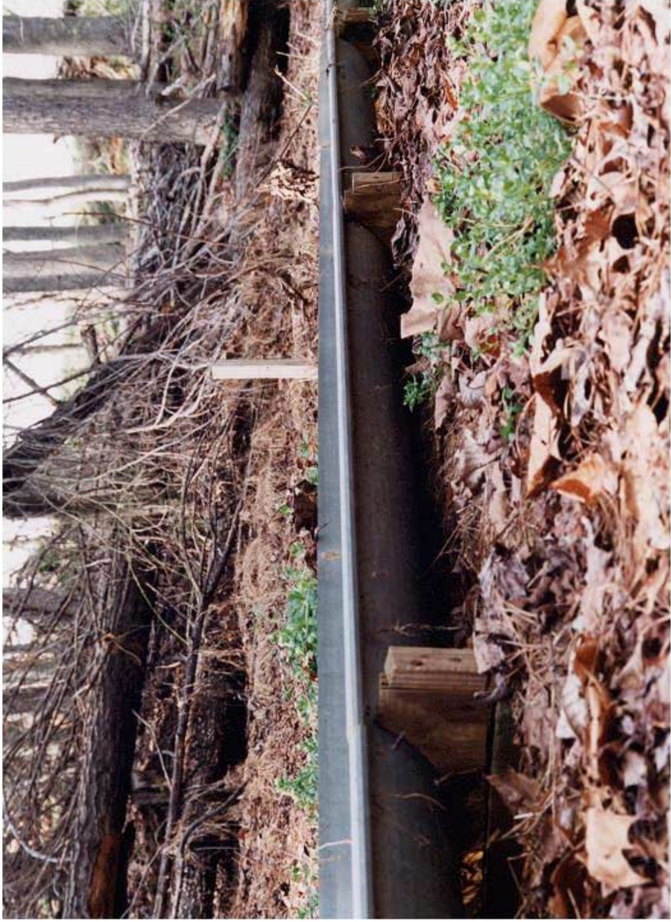
Figure 6. Level spreader made from galvanized gutters installed at the Pasture Site at the North Carolina State University Field Laboratory
