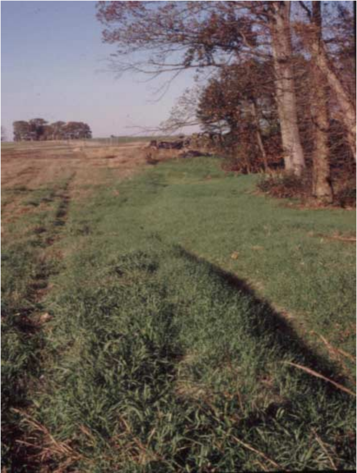
Figure 8. Trench and berm level spreader installed at the North Carolina State University Lake Wheeler Road Field Laboratory.
