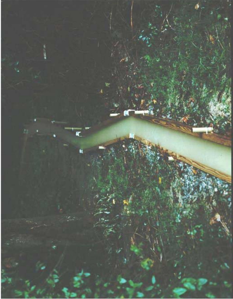
Figure 5. Level spreader made from treated wood installed at the Oxford Tobacco Research Station
