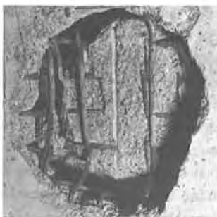
Figure 3. Foulness Test No 50 Front Face
