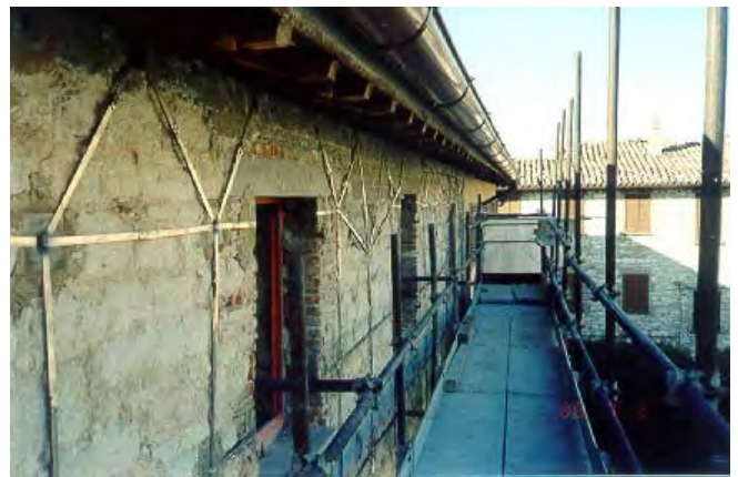
Figure 6: Application of the CAM method to the seismic improvement of a masonry apartment building at Sigillo (Perugia) (filmed during works in December 2000).
