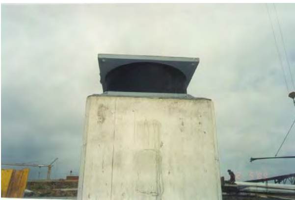
Figure 5: High damping rubber bearing just installed in the apartment houses of IERP at Città di Castello (Perugia), as filmed in May 2001.
