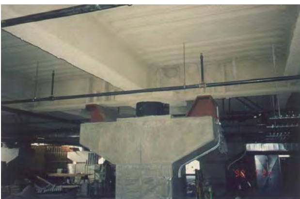
Figure 1: Seismic isolation system (rubber bearings) of the new Emergency Management Center of San Francisco, California, USA (filmed in July 2000).
