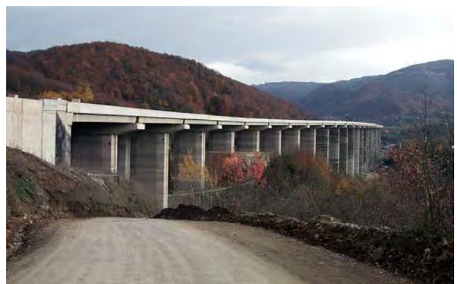
Figure 2: Viaduct of the Istanbul – Ankara freeway, provided with elastic-plastic dampers, which survived the 1999 earthquakes (filmed in May 2000).
