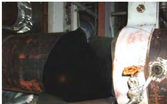
Fig. 1: Burst pipe in Mihama 3 NPP
