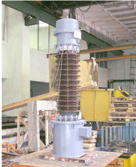
Fig. 7 Testing of voltage transformer
