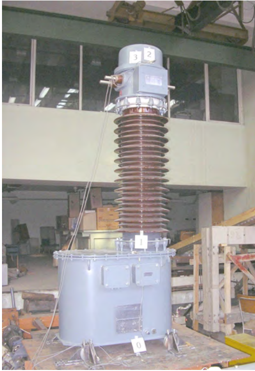
Fig. 8 Testing of combined transformer
