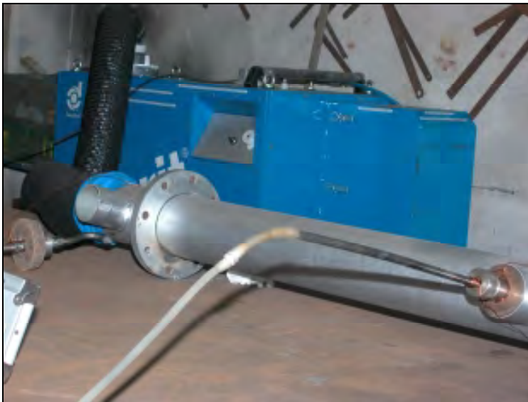
Fig. 6 Measurement chimney, with the derivation for the filtering device and the apparatus for the suction of smokes and for the absolute filter.
