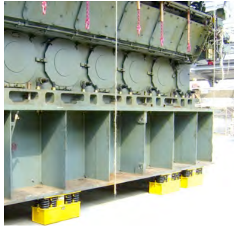
Figure 1. Emergency Diesel Generator with Base Control System.
