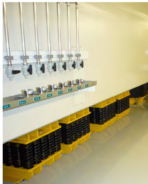
Figure 5. 3-D Base Control System below a spent fuel pool in a high seismic zone.
