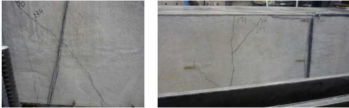
a) Shear cracks for out of plane load of 234 kips
