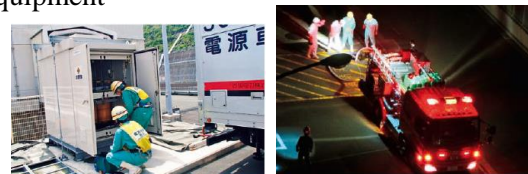
Figure 5. Left: Status of training on installation work at SA equipment installation port and Right: Status of night-time work training
