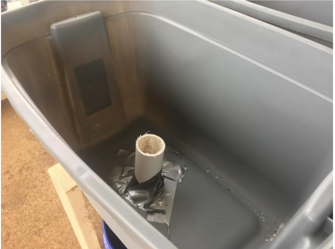
Figure 2. Outlet chamber in bottom of bioretention cell is shown.
