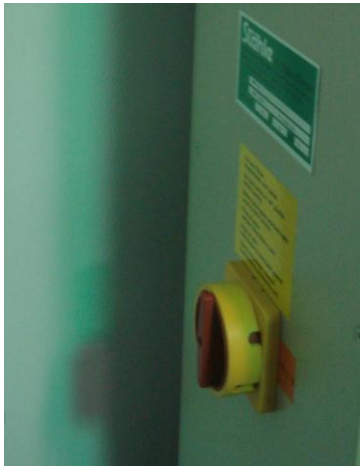
Figure 3.13: Electric panel switch
