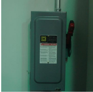
Figure 3.12: Power supply switch
