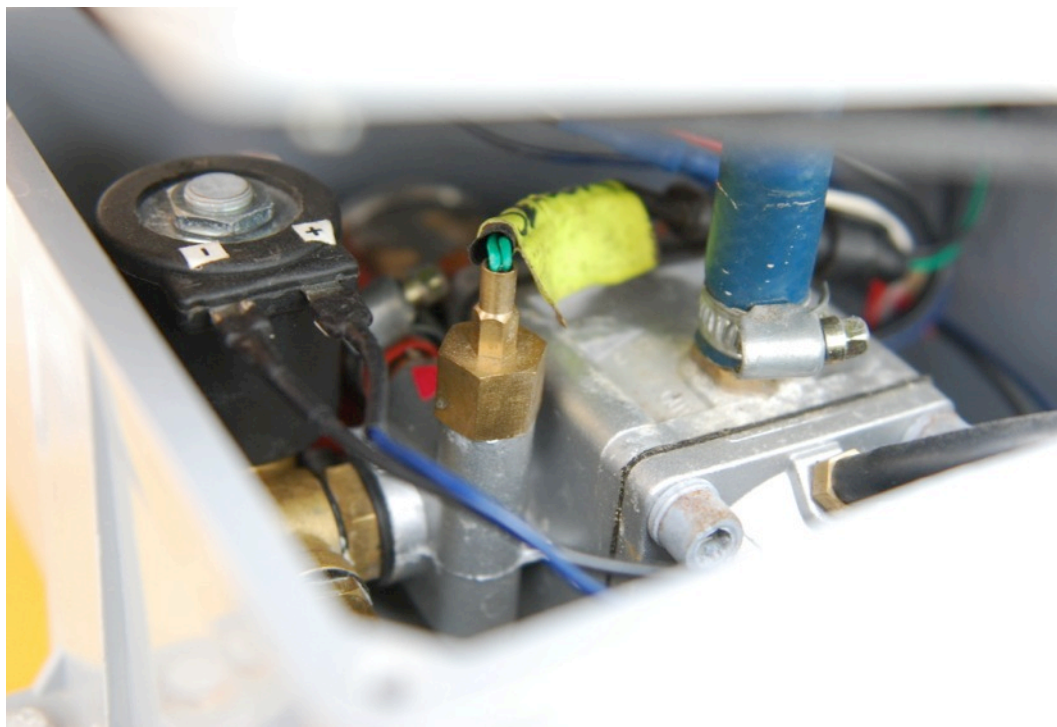
Figure 18 - CNG pressure reducer and electro-valve system
