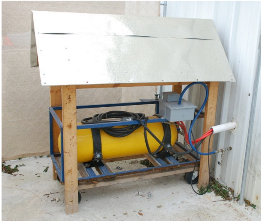
Figure 16 - CNG tank in enclosure
