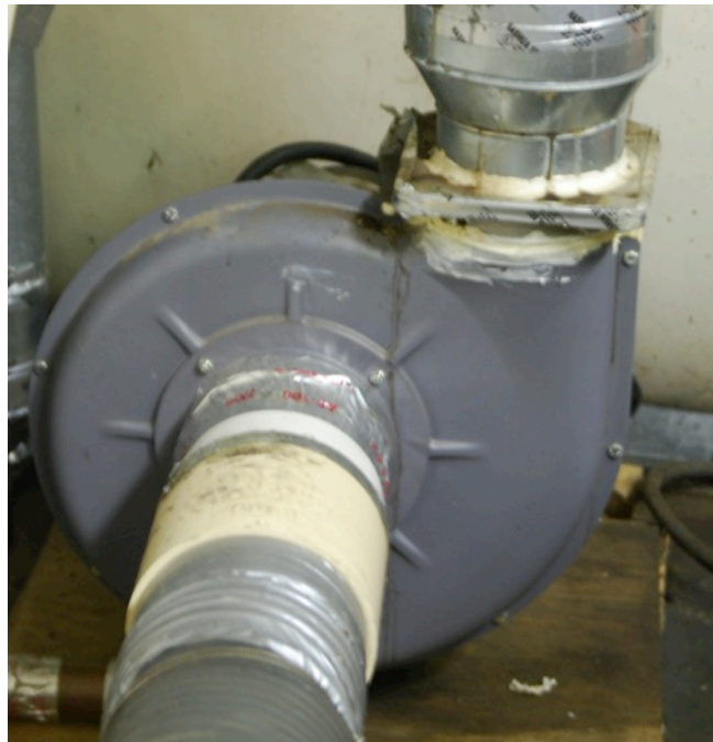
Figure 11 - Exhaust removal blower
