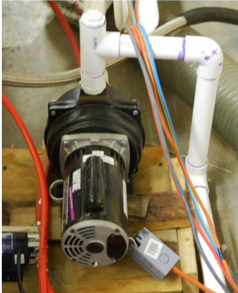
Figure 5 - Wayne 1.5 hp main feed water supply pump
