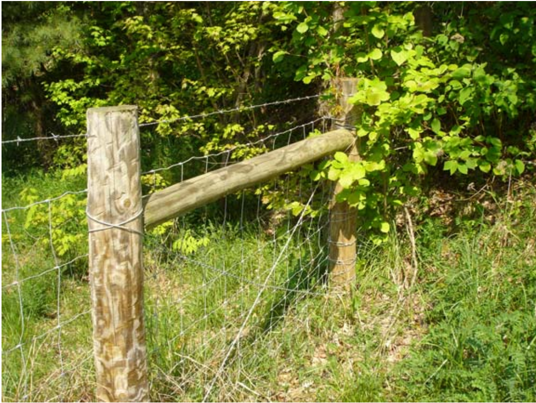
Figure 6. A more detailed view of the right-of-way fencing. It is constructed of welded wire, barbed wire, and wooded posts.
