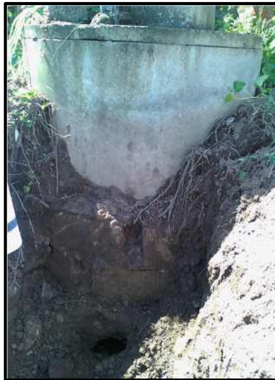
Figure A.5 Pit latrine that must be accessed from the side because of a design not compatible with pit emptying (Still and O’Riordan 2012).
