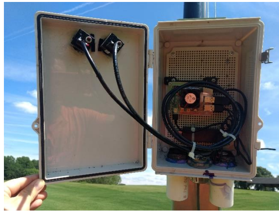
Figure 2.2: Camera system electronics installation
