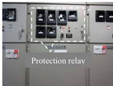
Figure 2. Metal-clad switchgear protection relay before digitalization.
