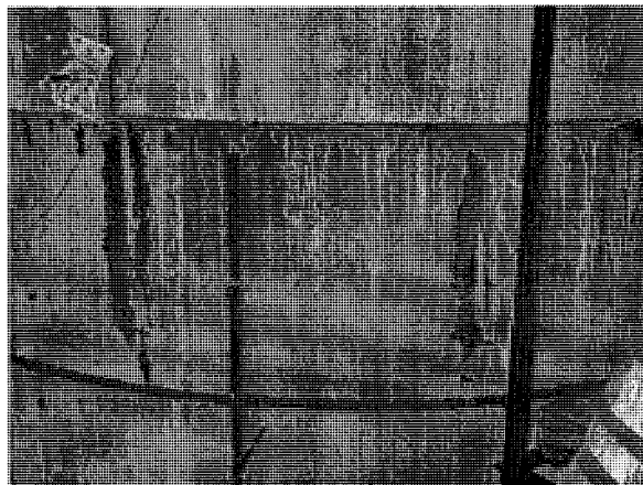
Slowly Starting Leakage at the Top of the Cylindrical Wall at 1.7 MPa
