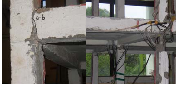
Fig 11 Damage patterns observed at PGA = 0.6g and 0.7g
