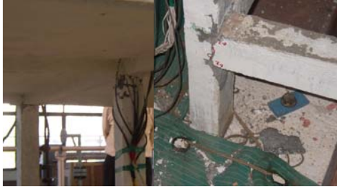
Fig 10 Damage patterns observed at PGA = 0.5g
