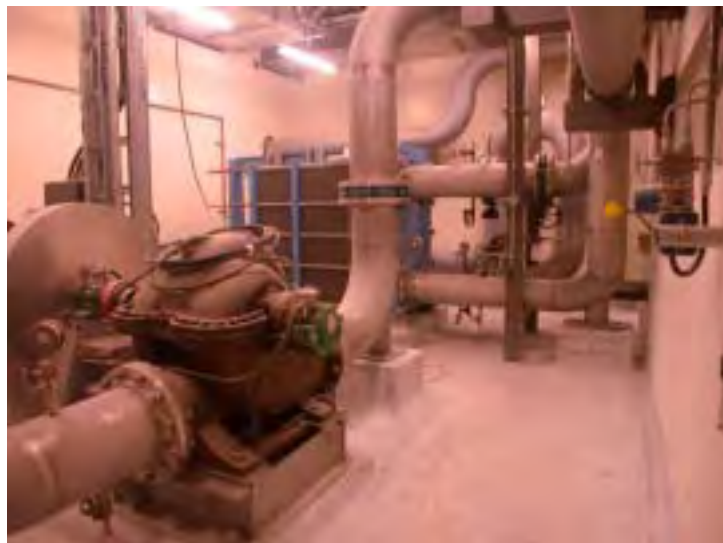
Figure 12 – Primary Cooling System Pump and Heat Exchanger
