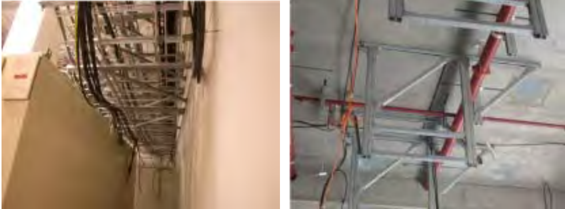
Figure 20 – Cabletrays and supports with lateral and longitudinal bracing
