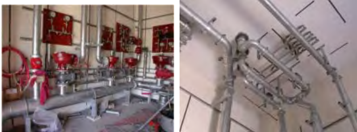
Figure 17 – Fire System Valves and Piping
