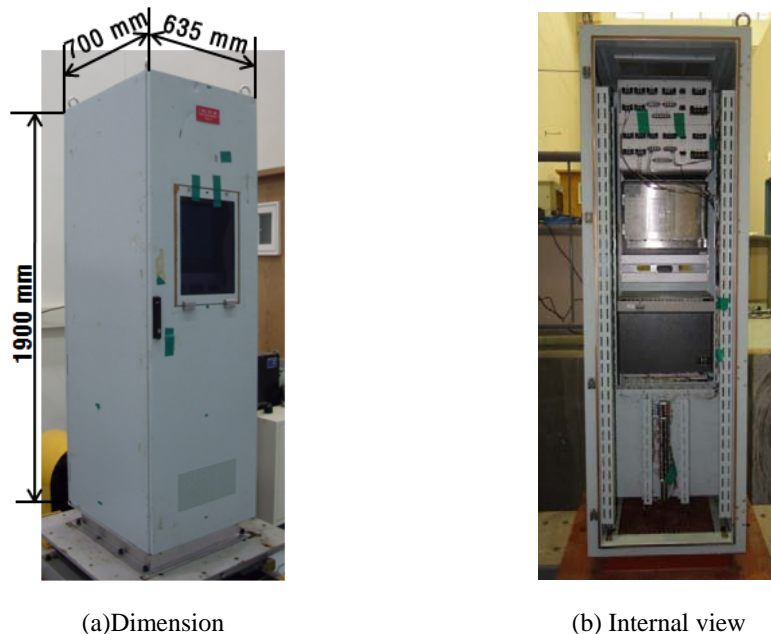
Figure 1. Test cabinet on the mounting fixture
