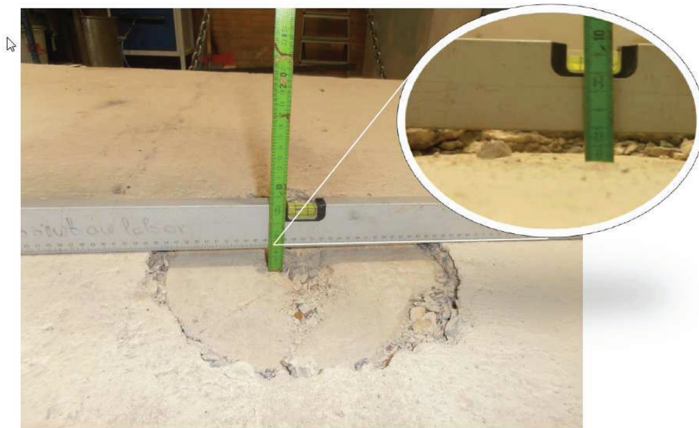
Figure 5: Penetration effects on the impacted face of slab DL1
