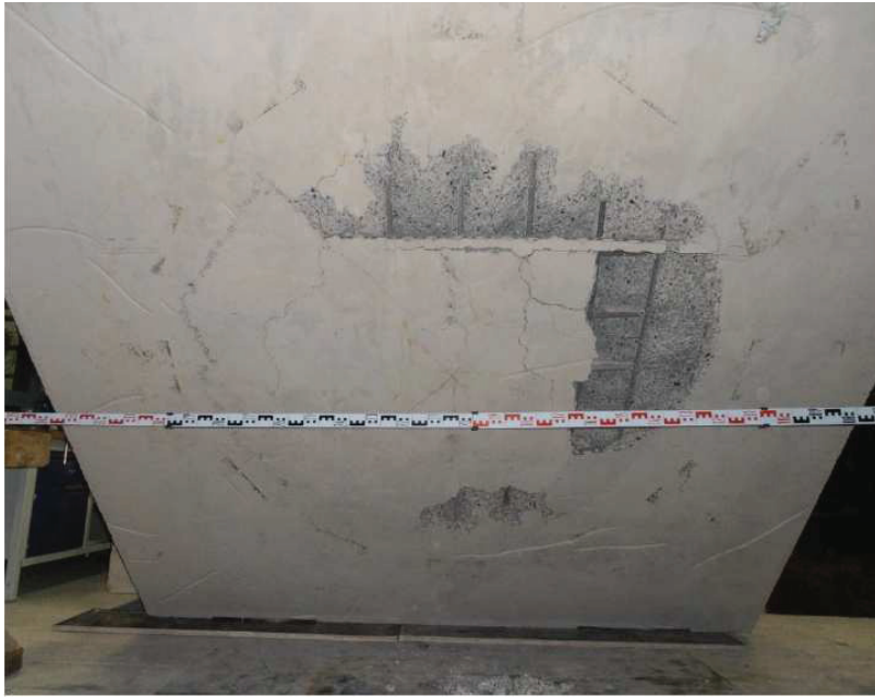
Figure 4: Bottom face of Slab DL1 with visible punching cone diameter of 1,50 m
