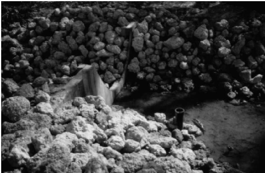
Fig. 1.4. Two prominent features of a typical retention device (Hunt and Doll, 2000). First is the principal spillway. In this photograph the principal spillway is the wooden weir. The second is a drawdown device. In this case the small riser pipe has holes drilled into it behind the protective rocks. The difference in elevation between the drawdown device and the principal spillway dictates the wetland's temporary storage volume.
