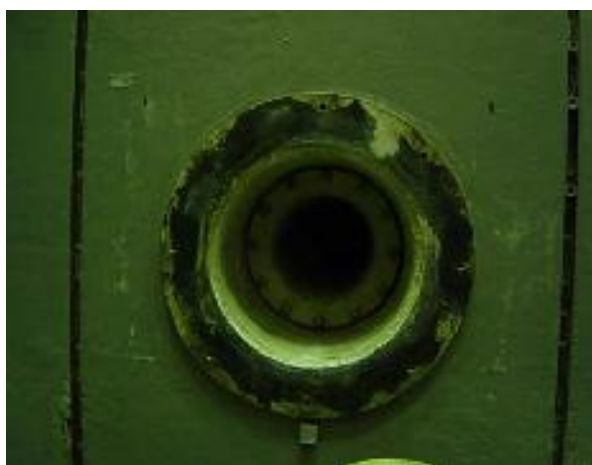
Fig. 3.16. Bare beam tube #5 of the reactor.
