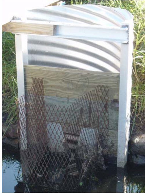
Figure 3.8 Water control structure with 30° V-notch weir.
