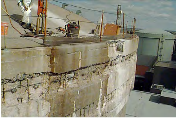
Figure 5 Condition of the Ring Beam Before Repair
