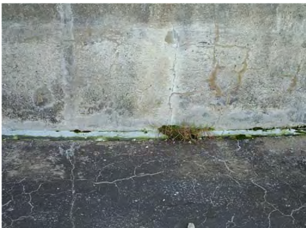
Figure 9 Deterioration of Sealant at the Bottom of R/B
