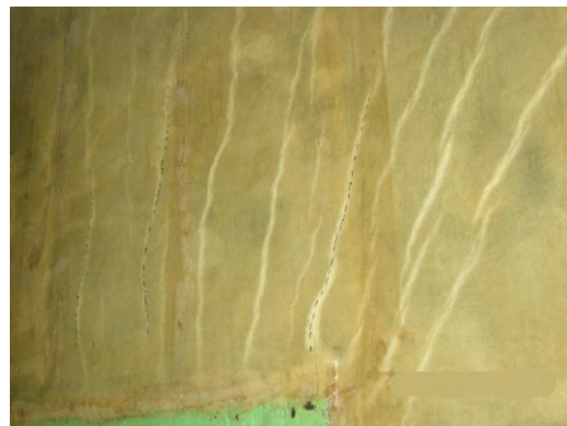
(b) Cracking observe after experiment at upper corner of MAL
