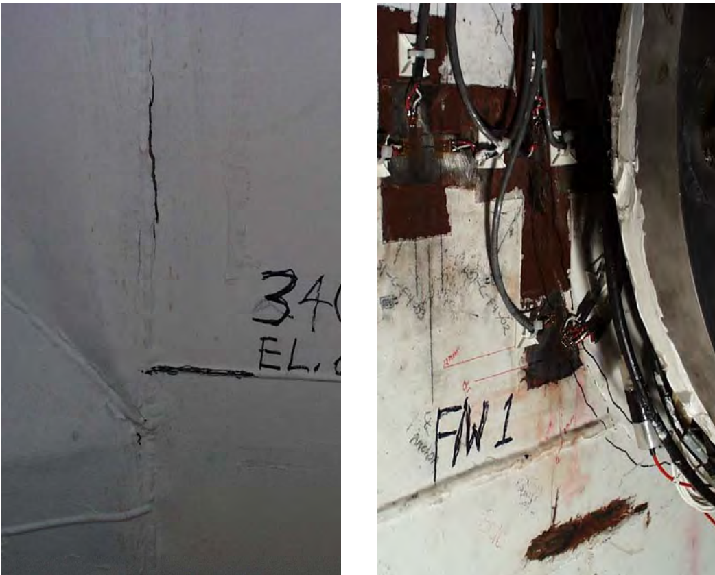
Figure 18 Liner Tear at Locations 15 (Equipment Hatch) and 3 (Feed water Penetration)
