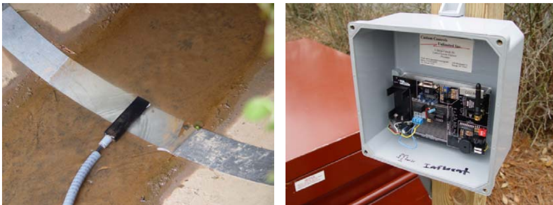
Figure 11 a and b Low profile Area-Velocity probe at Outlet and Wireless Sampler Triggering Device at Pierson Pond.
