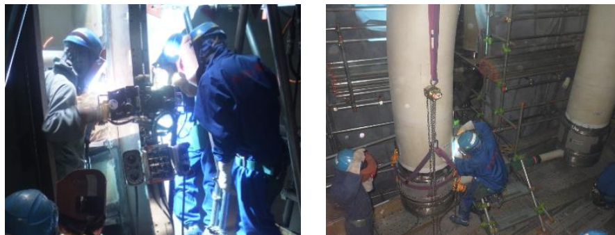
Figure 5: Example of modification work in progress (Left: suppression chamber, Right: vent system)
