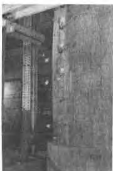
Figure 3. Crack Pattern and Bulging of Wall at 130 psi (0.90 MPa)
