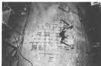
Figure 5. Failure Zone, Note Anchorage Distress, Broken Reinforcement and Tendons
