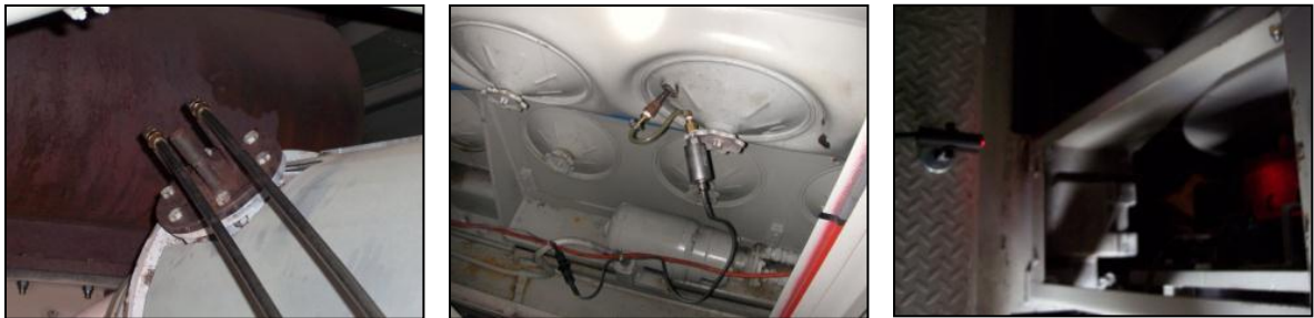
Figure 2-3: Installation of Sensors on an F59PH Locomotive Prime Mover Engine (a) exhaust sampling port and metal tubes; (b) manifold absolute pressure (MAP) sensor; (c) RPM sensor
