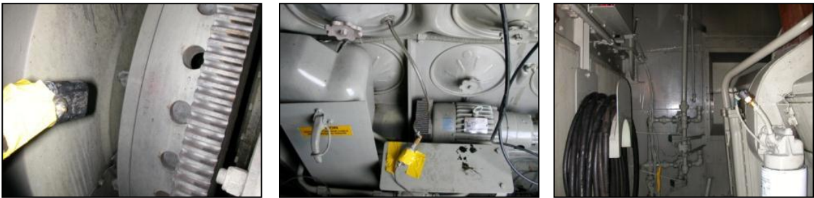
Figure 2-6: Installation of Sensors on an F59PHI Locomotive Prime Mover Engine (a) RPM sensor; (b) manifold absolute pressure (MAP) sensor; (c) intake air temperature (IAT) sensor
