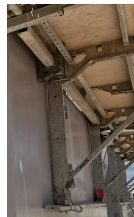
Support to working platform
