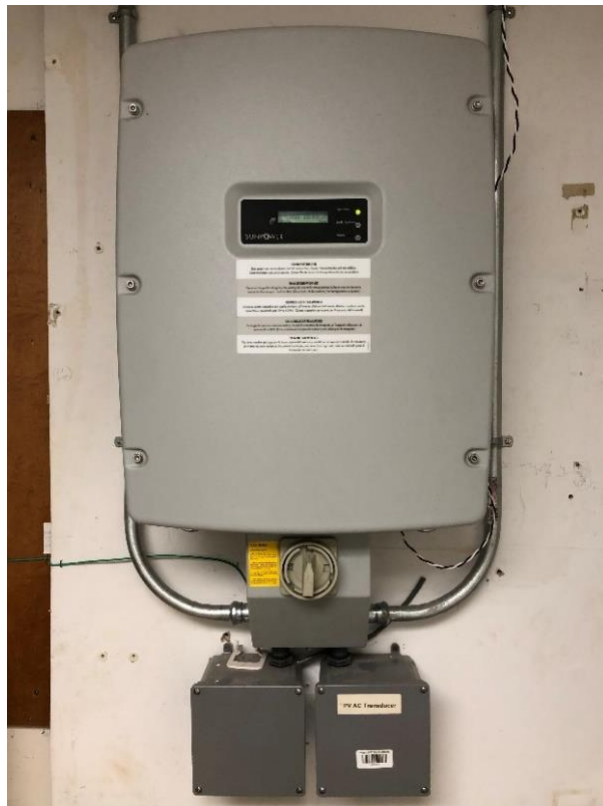
Figure 1.2: The house inverter and AC disconnect.
