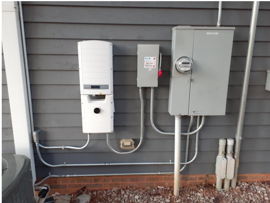
Figure 1.6: The garage inverter, AC disconnect, utility meter, and circuit breaker box.
