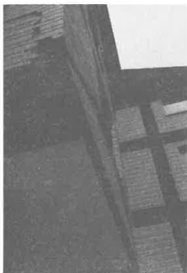
Fig. 9. II) A common type of damage resulting from brick infill panels not properly tied to structural frame.
