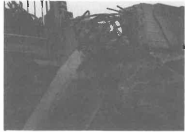
Fig. 4. I) Loss of bonding between steel and concrete in a column-beam connection. The earthquakes show that confidence in the use of high bond deformed bars is not completely justified.
