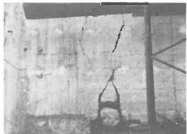
Fig. 6. IV) Failure of longitudinal steel in a beam. This type of damage is much less common than brittle type failure of heavily reinforced concrete.
