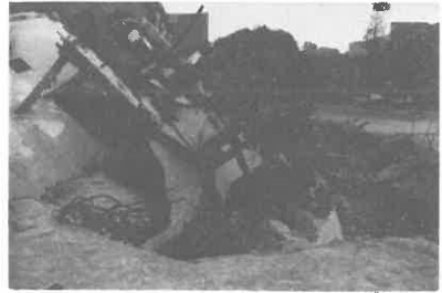
Fig. 12. IV) A spectacular example of foundation settlement caused by flow of clayey soil.
