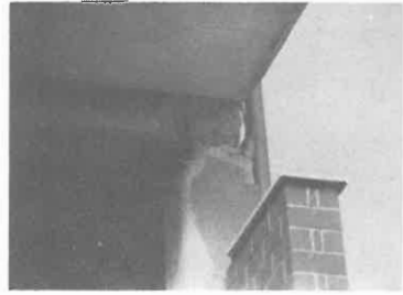
Fig. 3. I) Effects of lack of ties in a column-beam connection.
