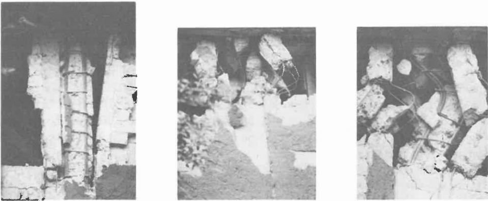
Fig. 1. IV) An ideal sequence shows an usual collapse mechanism in columns without sufficient ties.
