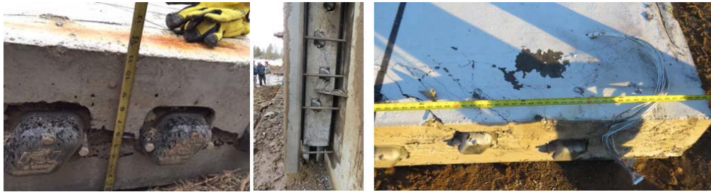
Figure 4. Through-thickness crack at the anchorages of the pre-stressing cables and cracked area at the edges of slab in Test 1
