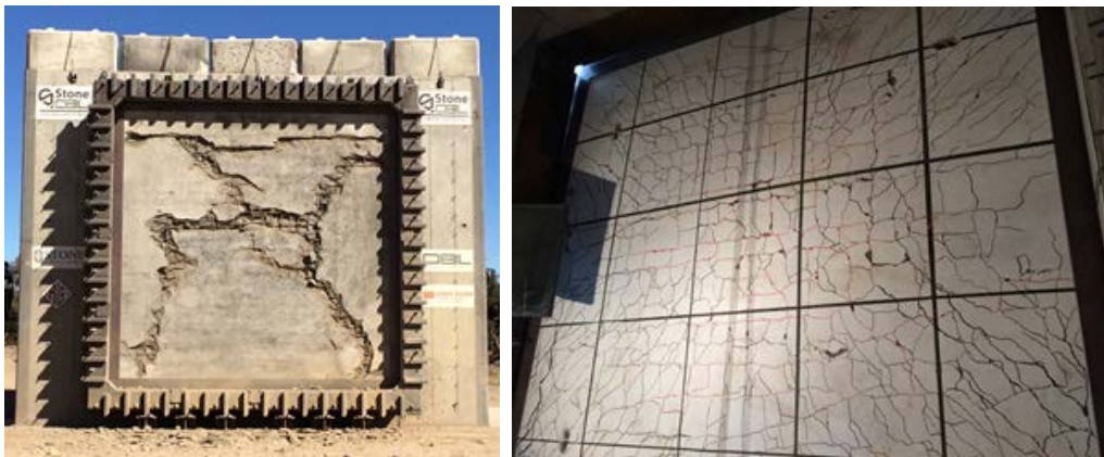
Figure 6. Front and rear side of the slab after Test 2b
