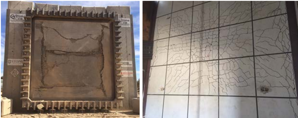
Figure 8. Front and rear side of the slab after Test 3
