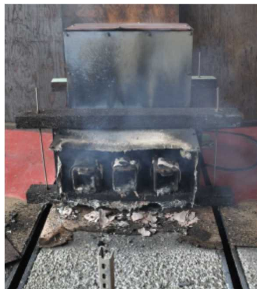
Figure 1. Bus Duct damage [9]
