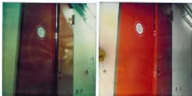
Figure 3. Fire door damaged by HEAF (from outside the room) [4]
