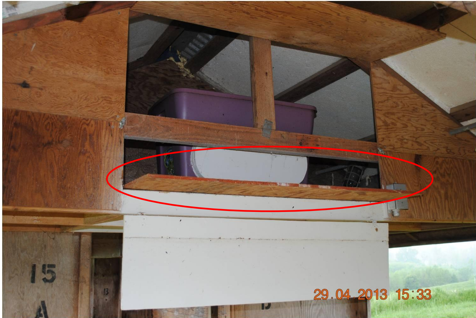
Figure 2. External view of one of the attics with both doors open. The removable floor panel is partially removed and enclosed within the circle.
