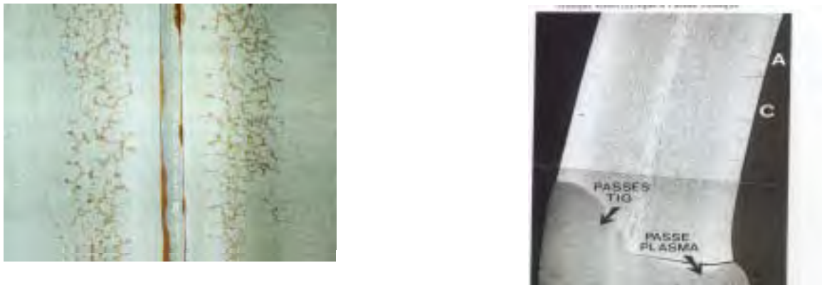
Figure 1: Typical cracks observed in the mixing zone of RHR..
