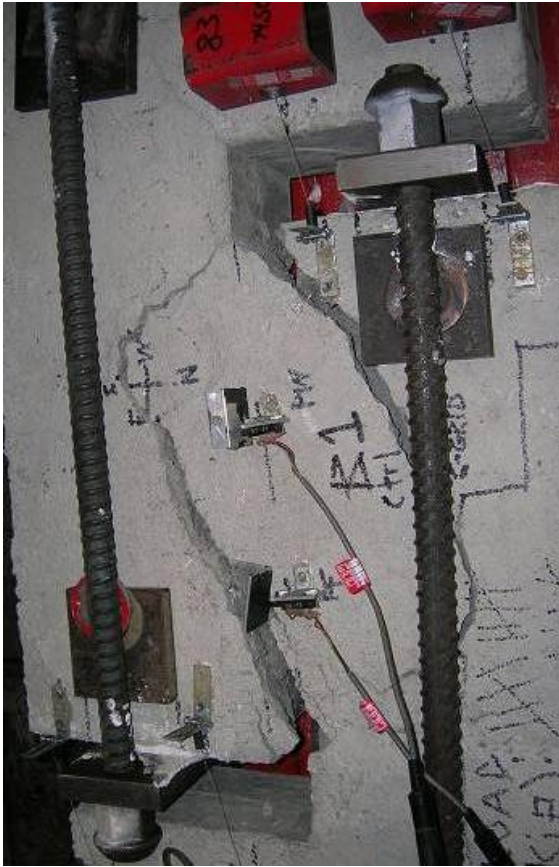
(a) Shear/Flexure Cracking
