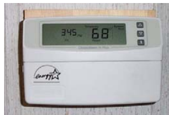
Figure 5.3.1.3: Installed Programmable Thermostat
