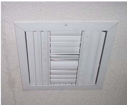
Figure 5.3.2: Closed Vent in the Experimental Classroom
