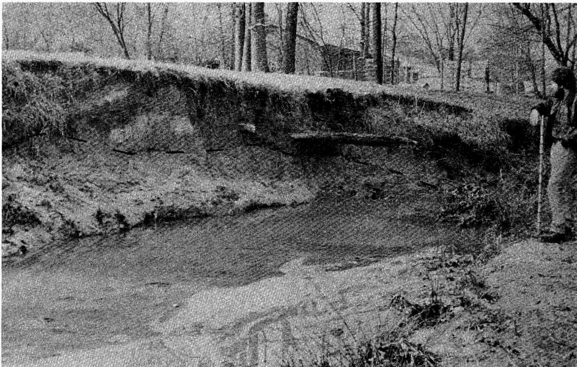
Fig. 5 Fill Overlying Gray Sediment. Dashed line on photo is at base of fill. Briar Creek at Plaza Road, Charlotte.
