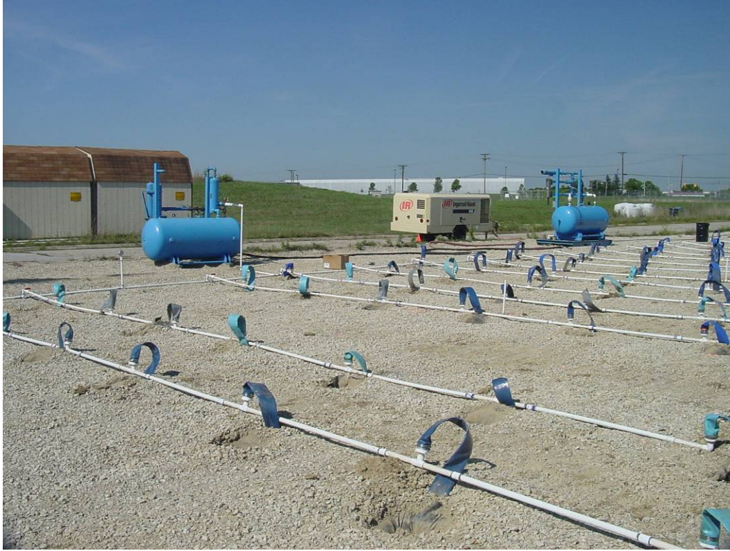
Figure 6. Photograph of Surface of Typical WIDE System Implementation on Contaminated Site
