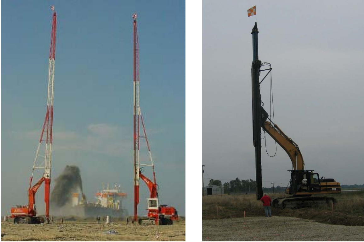
Figure 3. (a) Installation of PVWs Using Mandrels Mounted to Two Large Cranes and Excavators (Courtesy Cofra). (b) Installation of PVW Using Mandrel Mounted Excavators (Courtesy Nilex)
