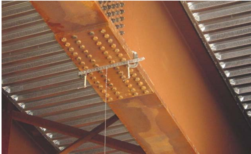
Figure 3-10 C-Clamps and Steel Angle Connected to the Bottom Flange of the Girder
