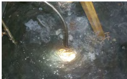
FIGURE 3.2 – Submerged wet welding inside a tank open electric arc is illustrated. (Note the welding fumes).
