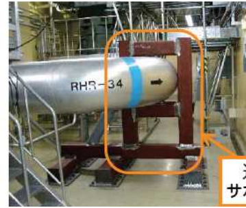
(additional piping support)
