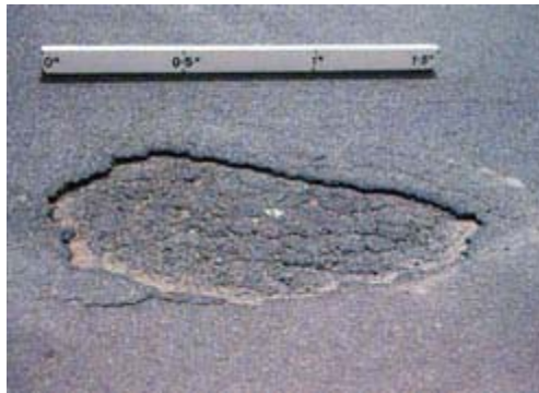
Figure 1-2 Delamination, exposure of underlying layer
