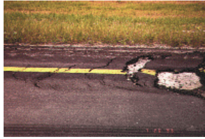
Figure 1-1 Delamination of surface course
