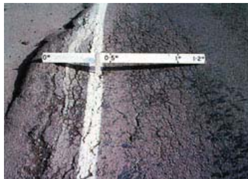
Figure 1-3 Distortion and shoving, deformation of surface layer under load
