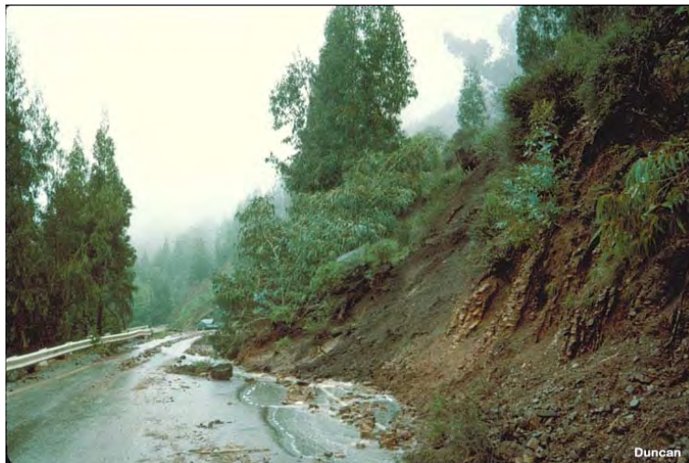
Figure 4: Effects of Unstable Soil Slope
