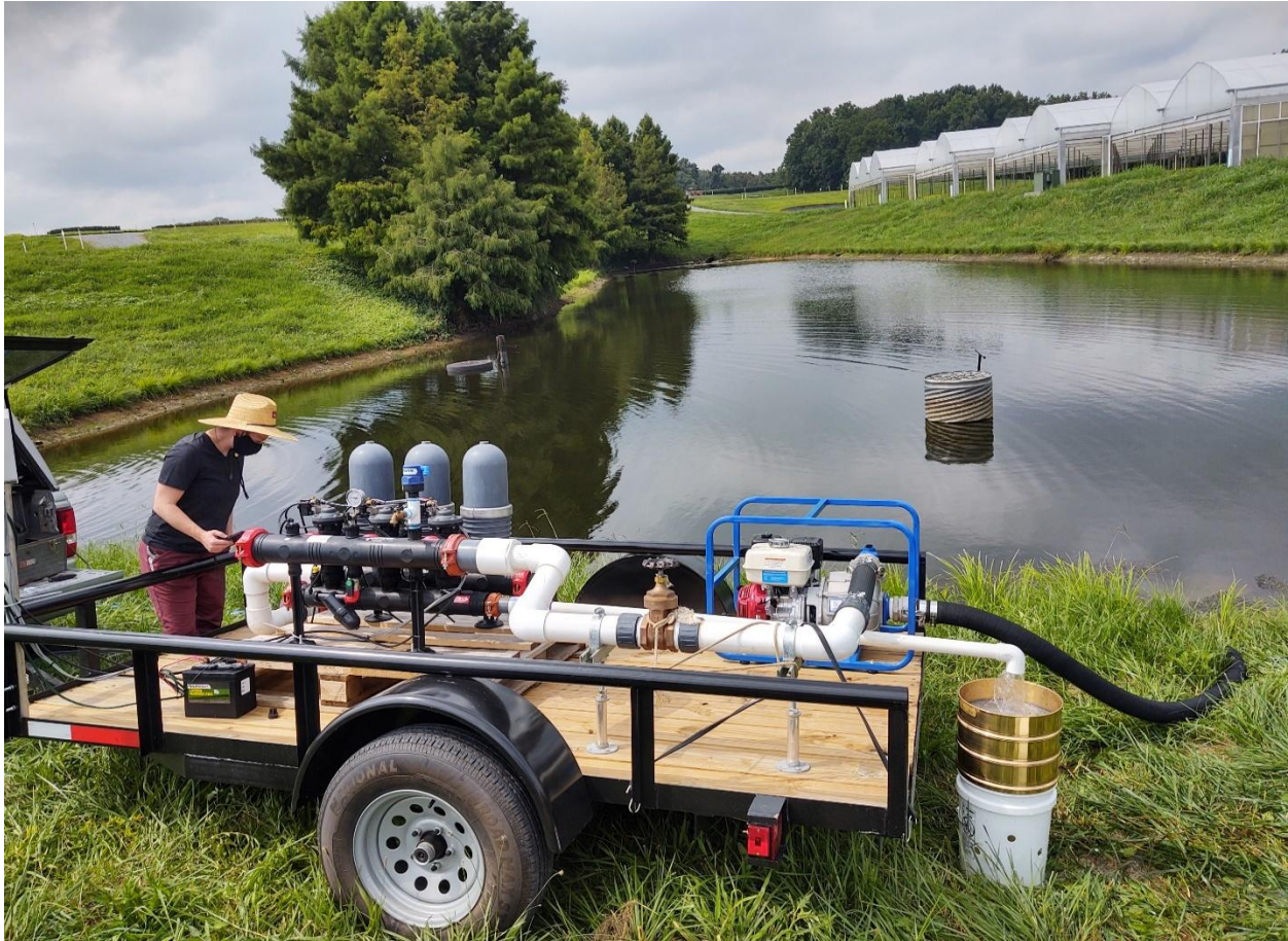
Figure C.1. Experimental setup at a container nursery of the pumping system used for irrigation filtration experiments. The backflow discharged from a PVC pipe is directed through a series of three sieves to capture filtrate samples. These sieves captured filtrate samples, while a 5-gallon bucket, with holes drilled to allow water passage, kept the screens off the ground.
