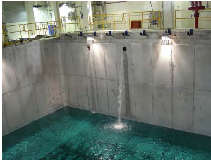
Figure 5 - Spent fuel bay filling with demi-water.
