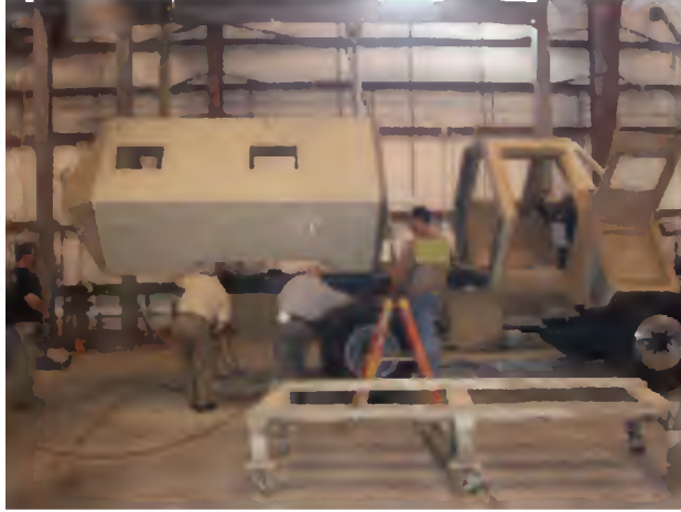
Figure 15. In the process of decking the vehicle with cab, body, & Front End Parts at Station 5.
